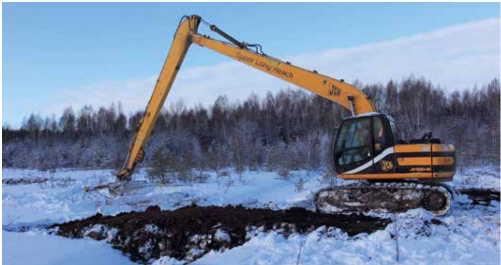
Figure 145. Installation of a peat dam in the Pūsčia area. Photo: Ž. Sinkevičius.
