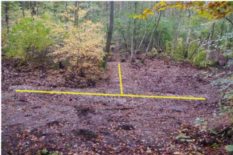
Figure 66. In the main direction of the water flow, the end of the BB-3's central drainage ditch and a T-shaped "catchment ditch" were filled with clay up to a depth of 2 m (October 2020). Photo: J. Etzold.
