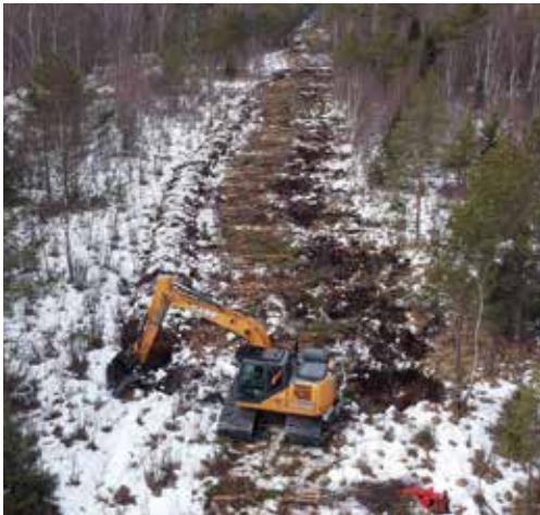
Figure 23. Construction of a peat dike running along the Piirsalu stream. Photo: R. Pajula.
