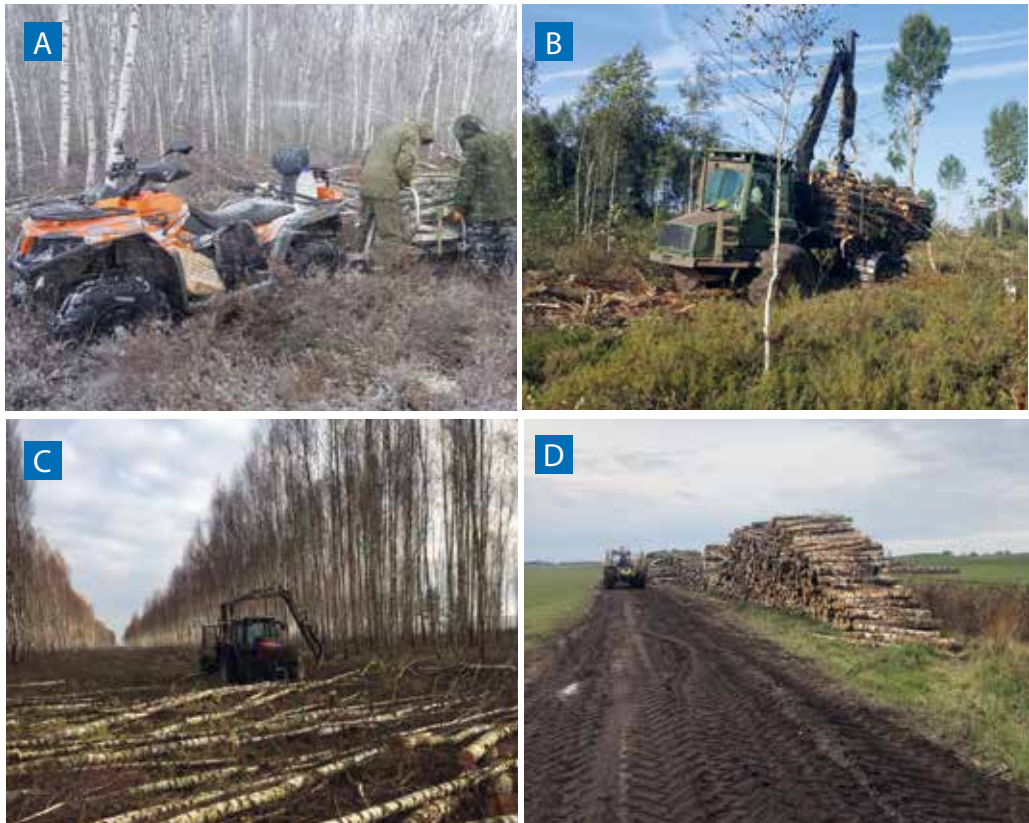
Figure 125. Removal of woody vegetation from the Amalva area: A – by light minitractor with a small trailer, March 2019; B and C – by heavy machinery (forwarders); D – timber yard on a roadside near the project area. Photos: Ž. Sinkevičius (A–C), N. Zableckis (D).
