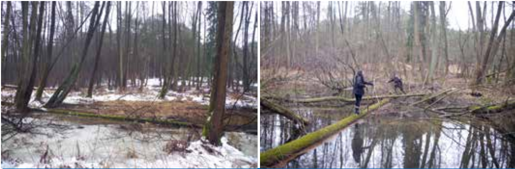
Figure 72. To increase the water level in the Pfauenfließ River, structures like logs, branches and soil material were placed in an irregular manner reducing the cross-section of the watercourse (February 2021). Photo: J. Etzold.
