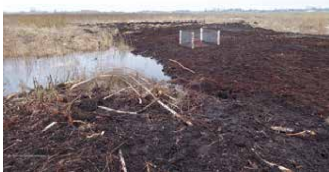
Figure 128. Dam with water outflow construction in Amalva peatland, March 2021. Photo: J. Sendžikaitė.
