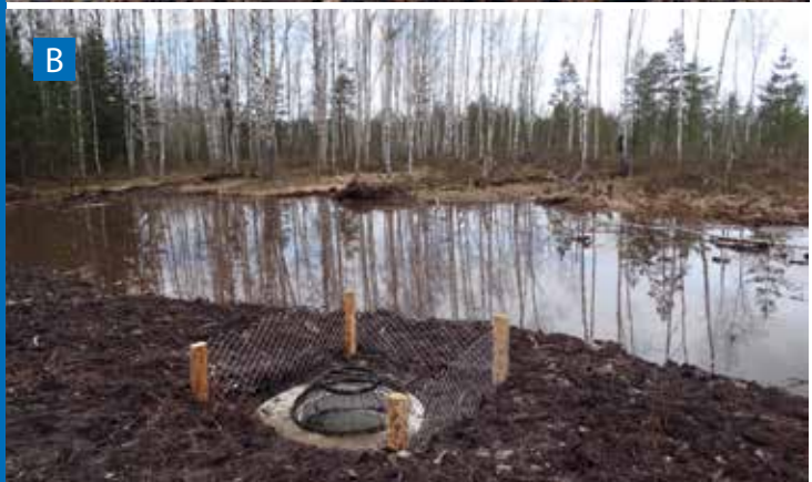
Figure 163. Installation of water outflow embankment (A) with a water outflow construction (B) in Sachara peatland, March 2020. Photo: L. Jarašius.
