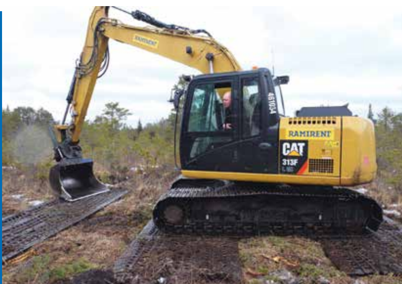
Figure 21. An excavator used for dam building. The paths for movement were first cleared of trees. Metallic footers help the heavy (15–20 t) machinery move on soft peat soil. Photo: R. Pajula.
