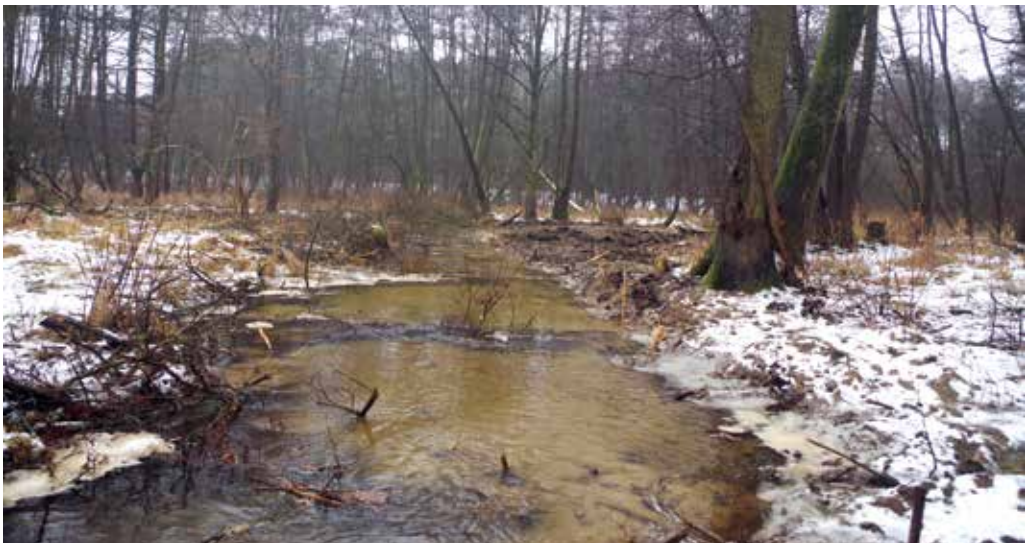
Figure 71. A view downstream along the bottom glide (work completed, February 2021). Photo: J. Etzold.
