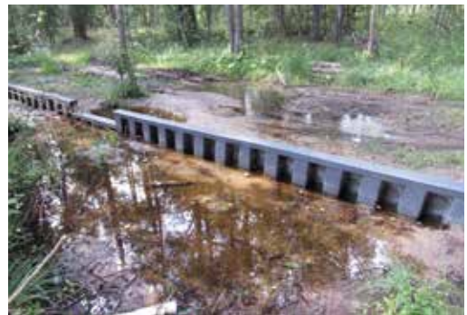
Figure 44. Plastic dam in the Engure restoration area in August 2021, more than half a year after building. Photo: A. Priede.
