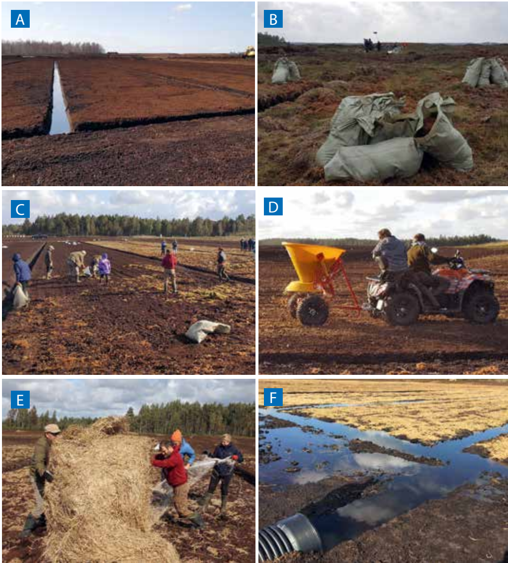
Figure 171. Reintroduction of peat-forming vegetation on peat fields in Aukštumala peatland, Lithuania: A – levelling of peat surface (April 2019), B – collection of donor material; (C) manual and (D) mechanized application of the donor material; E – straw mulching; F – flooded field covered with straw mulch (September 2019). Photos: J. Sendžikaitė, L. Šveistytė, Klasmann-Deilmann Šilutė.
