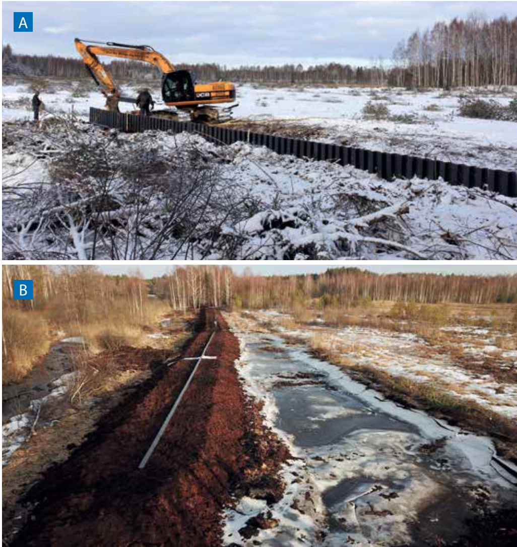
Figure 151. Protective peat embankments reinforced with plastic pile sheets. Construction process (A) and the installed embankment (B), February 2019. Photos: Ž. Sinkevičius.
