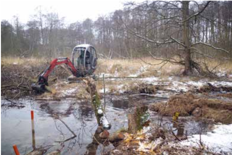
Figure 70. The excavator installing the so-called bottom glide shortly before the mouth of the Pfauenfließ into river Finow; woody materials, mineral soil and peat was used (February 2021). Photo: J. Etzold.
