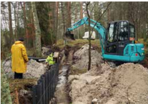
Figure 43. Installing the plastic piling in the Engure restoration area. Photo: M. Pakalne.
