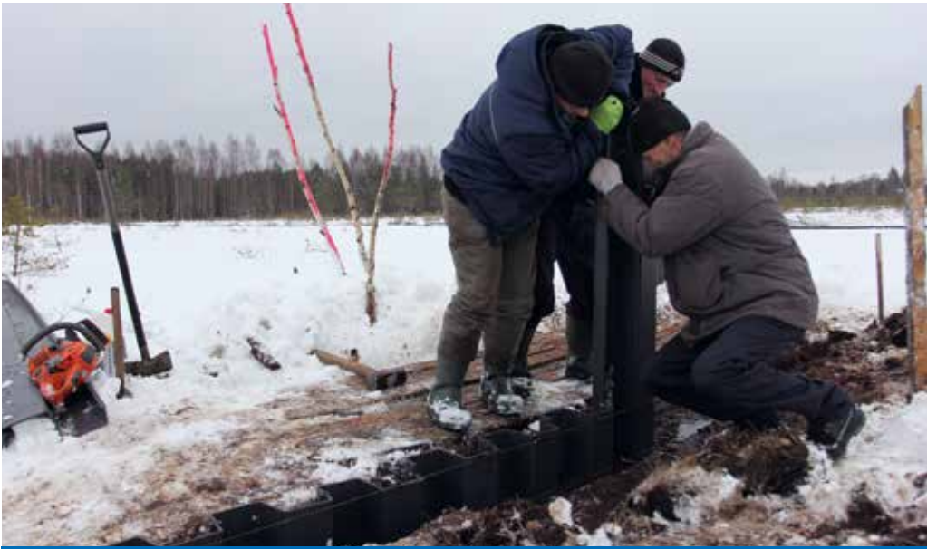
Figure 145. Installation of a peat dam in the Pūsčia area. Photo: Ž. Sinkevičius.
